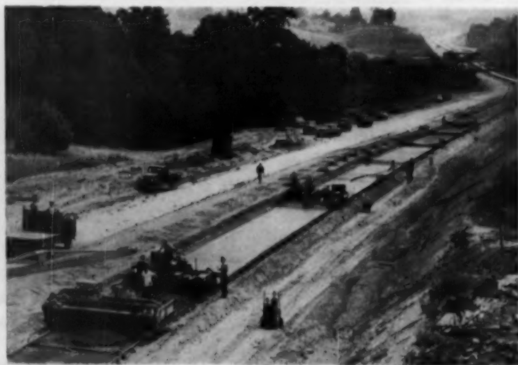
THE INCREASED use of the ride the rails road building technique directly parallels development of more modern road surfacing equipment.
